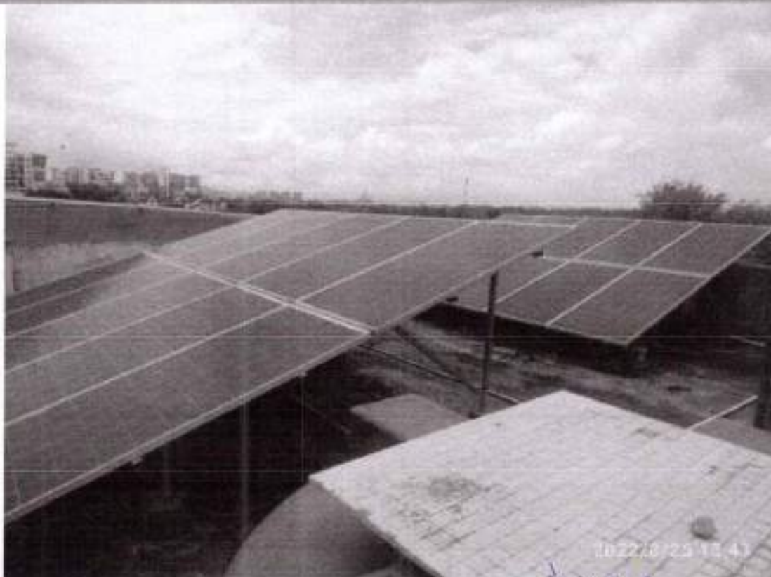
Solar Photovoltaic System- 15kWp
