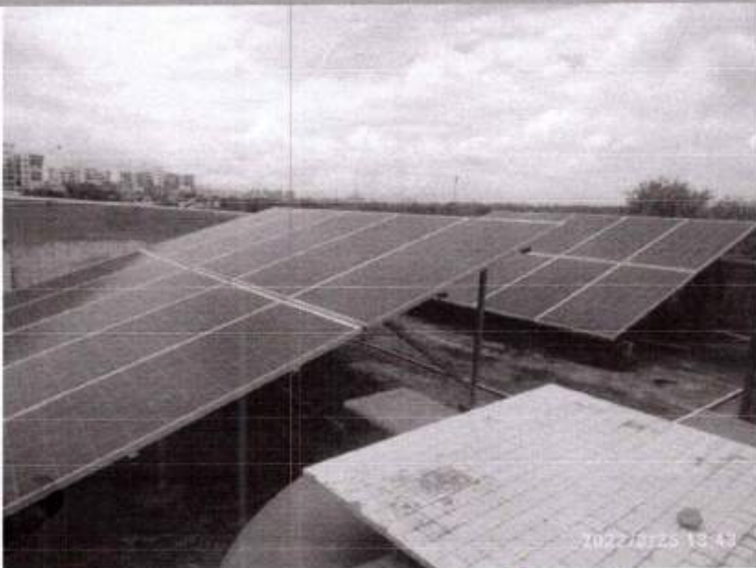
Solar Photovoltaic System- 15kWp
