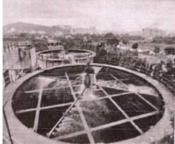
Pimple Nilakh STP has been quite rundown, with no security around tanks who have taken up the cause said the cement pipe bypassing treatment seen by MPCB officials was broken (R) a day after their visit
