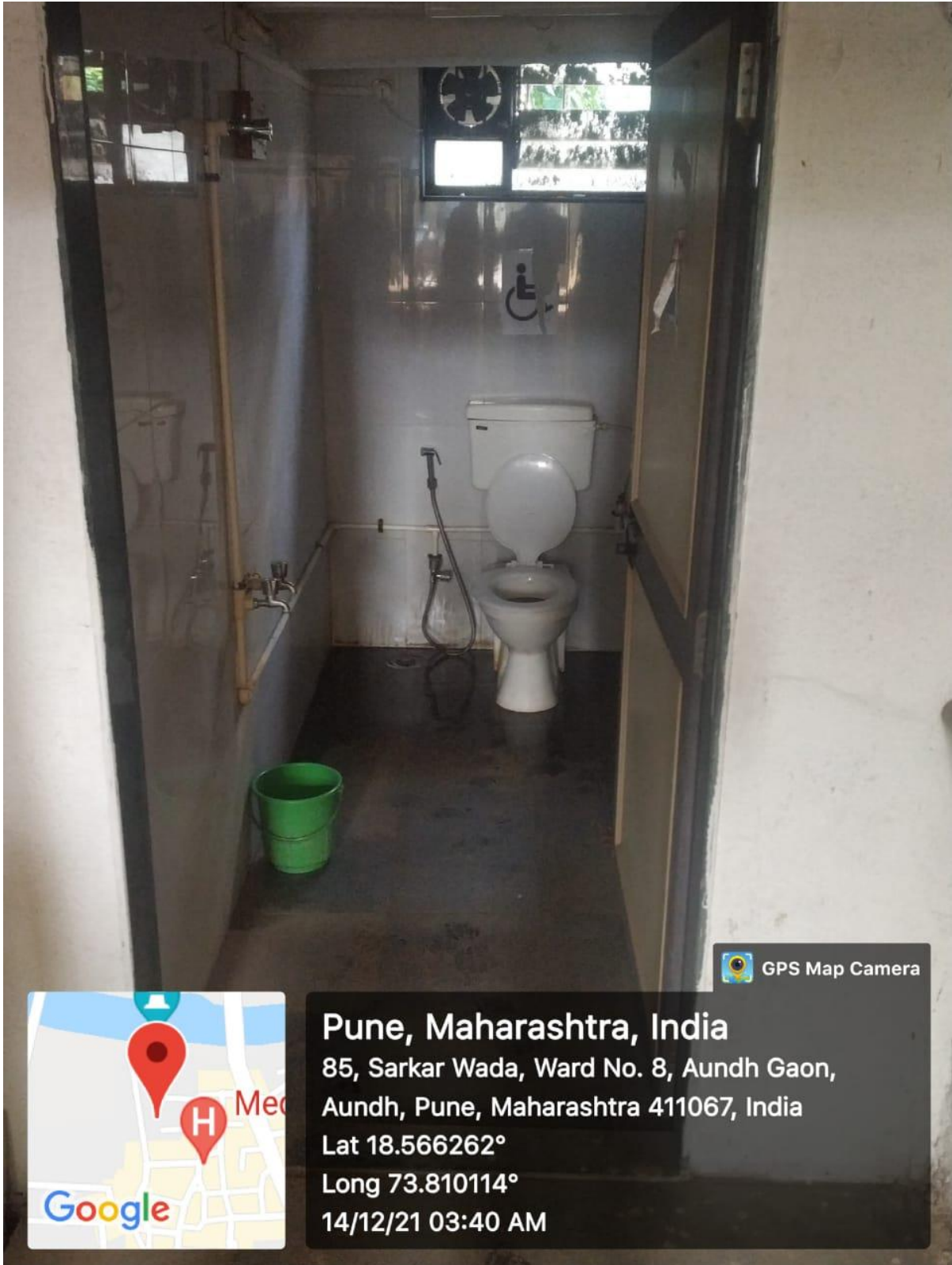
DISABLED FRIENDLY WASHROOM
