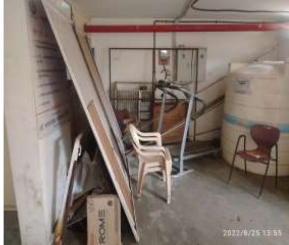
Unwanted waste material placed near electrical panel
