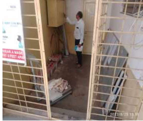
Unwanted waste material placed near electrical panel
