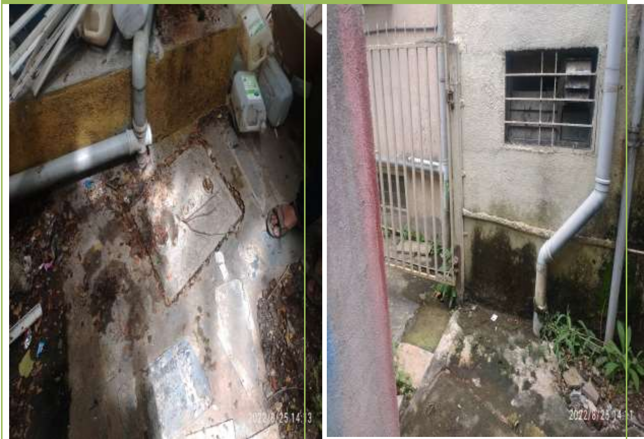
Rain water harvesting system in college premises
