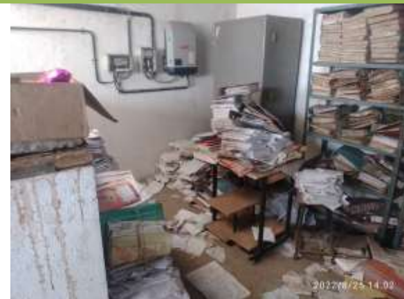
Unwanted waste material placed near electrical panel
