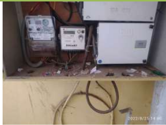
Electrical panel not clean
