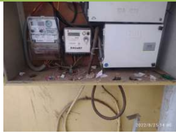
Electrical panel not clean
